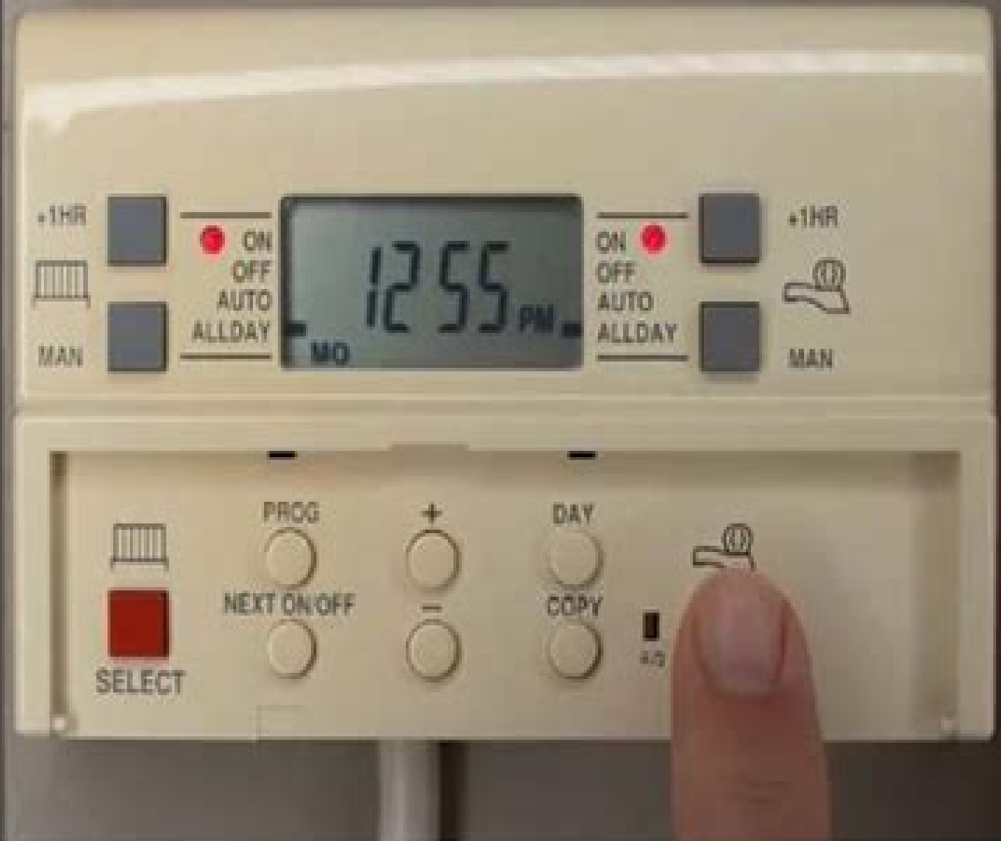
How to Set Digital Timer on Boiler?
