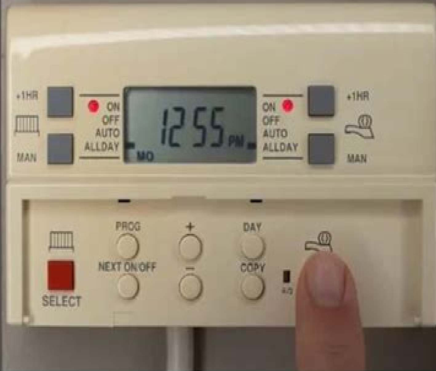
How to Set Digital Timer on Boiler?
