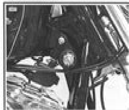
Figure 2-81. Control Cable Routing
