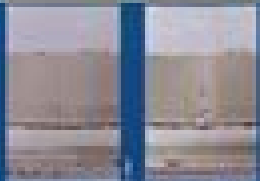
① Phenomenon: Flaking on Grooves, Spalls, Grooves, Ring Ribs ② Cause: Incorrect Handling during Assembly
