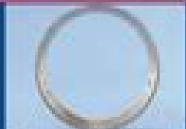
① Phenomenon: Flaking on Grooves, Spalls, Grooves, Ring Ribs ② Cause: Angular Assembly
