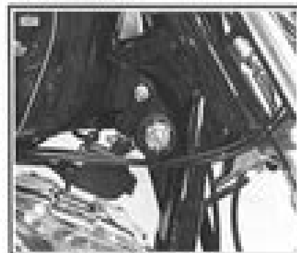
Figure 2-81. Control Cable Routing
