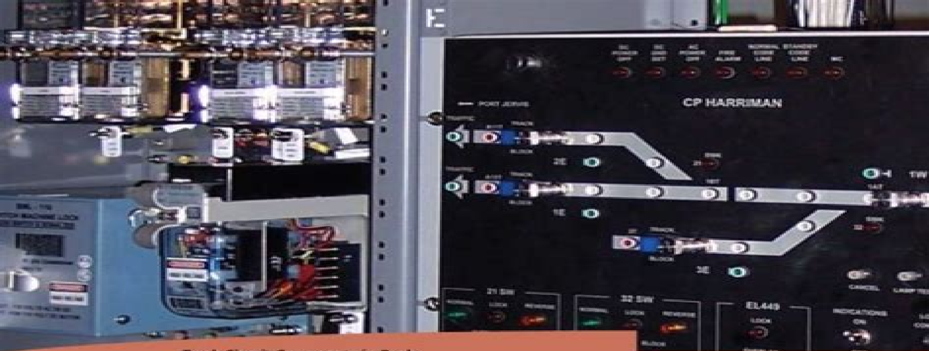
Track Circuit Components in Rack
